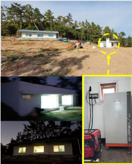
PV + Home ESS (5kW Inverter + BAT) + Diesel Generator
