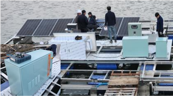
On Water Off-grid Hybrid ESS (옥천)
